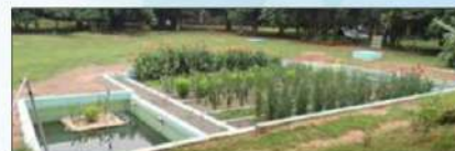
Constructed wetland for waste water treatment
